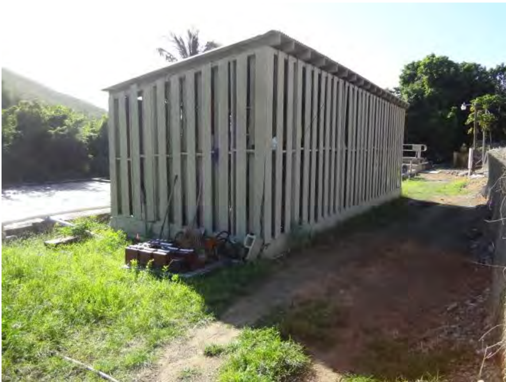
Wastewater Treatment Plant Pump Building – Soil Sample Location Near Pallet of Batteries on Ground
