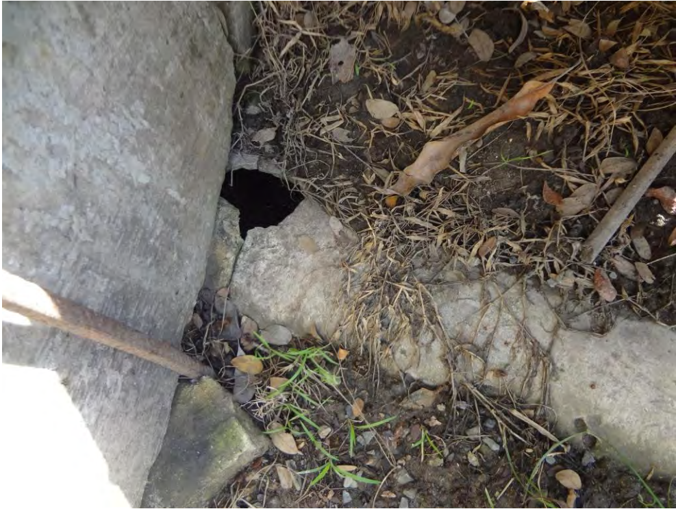
Grounds & Landscaping – Exposed Asbestos Pipe in Ground Near Equipment Maintenance Building
