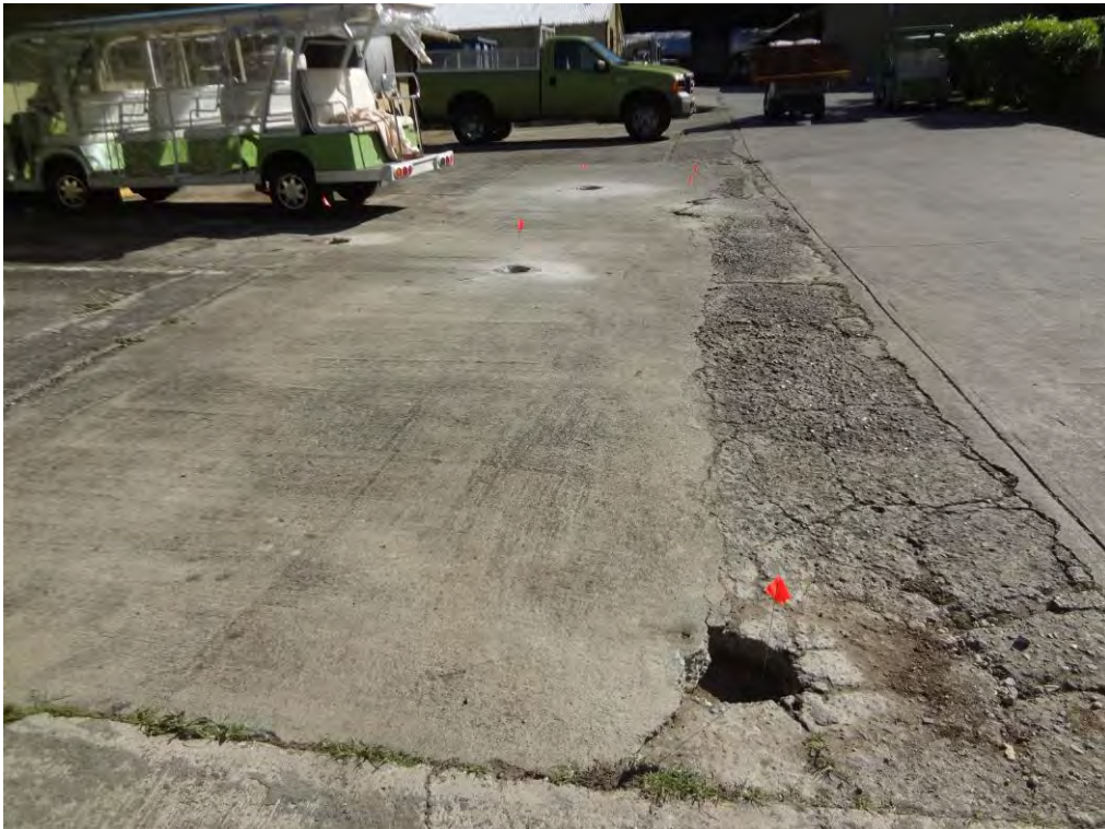
Boreholes Installed Through Pavement at Former UST Location – Borehole BH1 in Foreground
