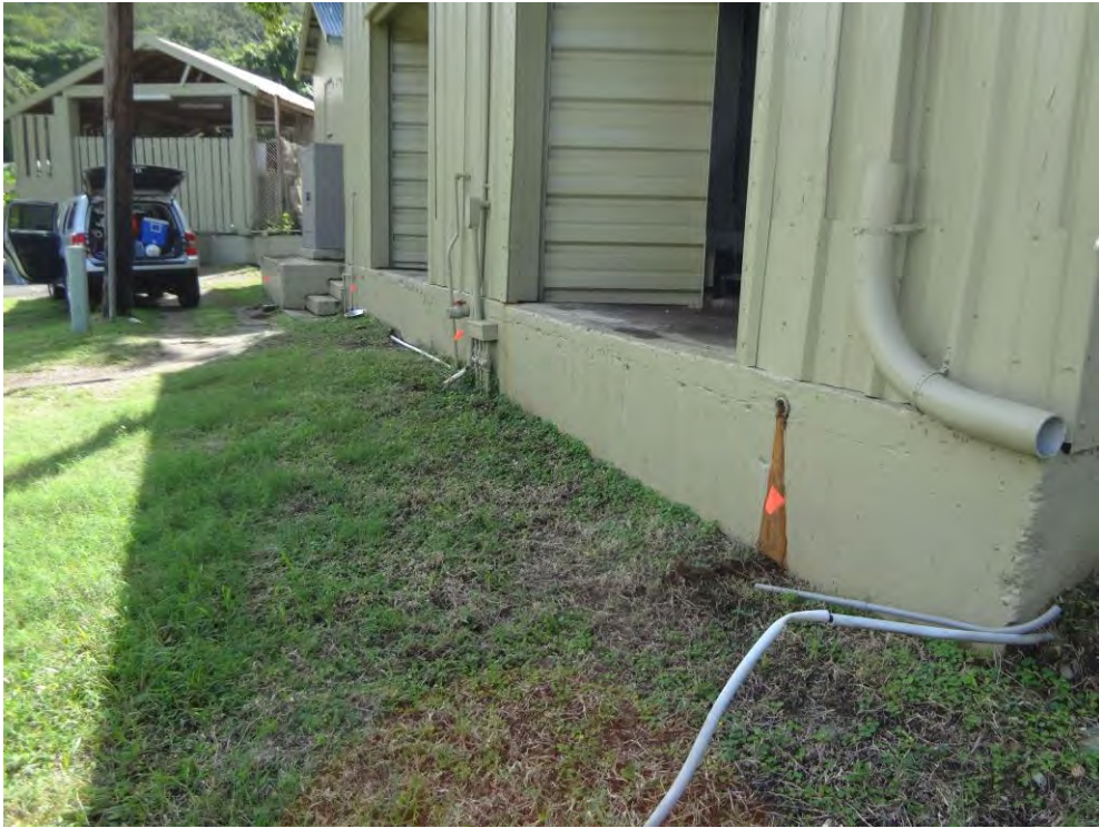
Northwest Side of Emergency Generator Building - Surface Soil Sample Locations
