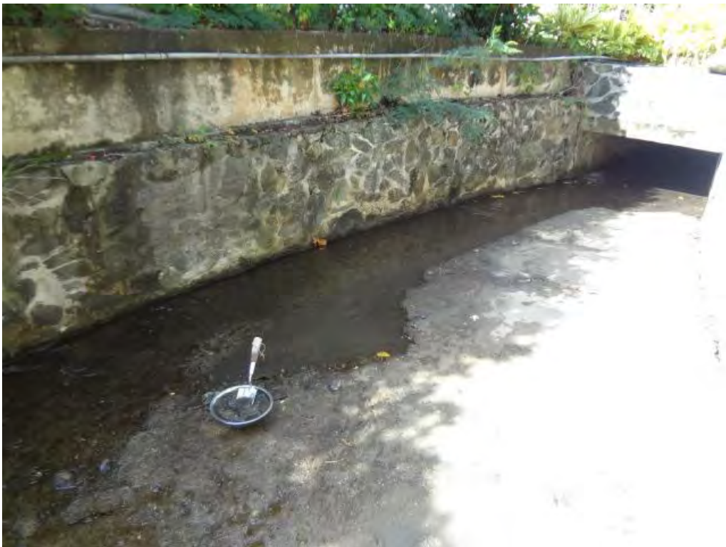
Paved Ditch Northwest of Engineering Area – Sediment Samples Collected in this Area
