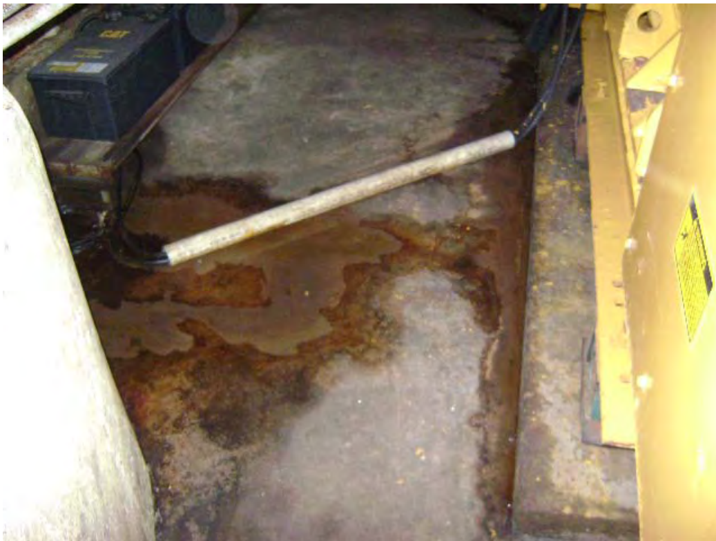
Oil & Batteries on Concrete Floor of Emergency Generator Building
