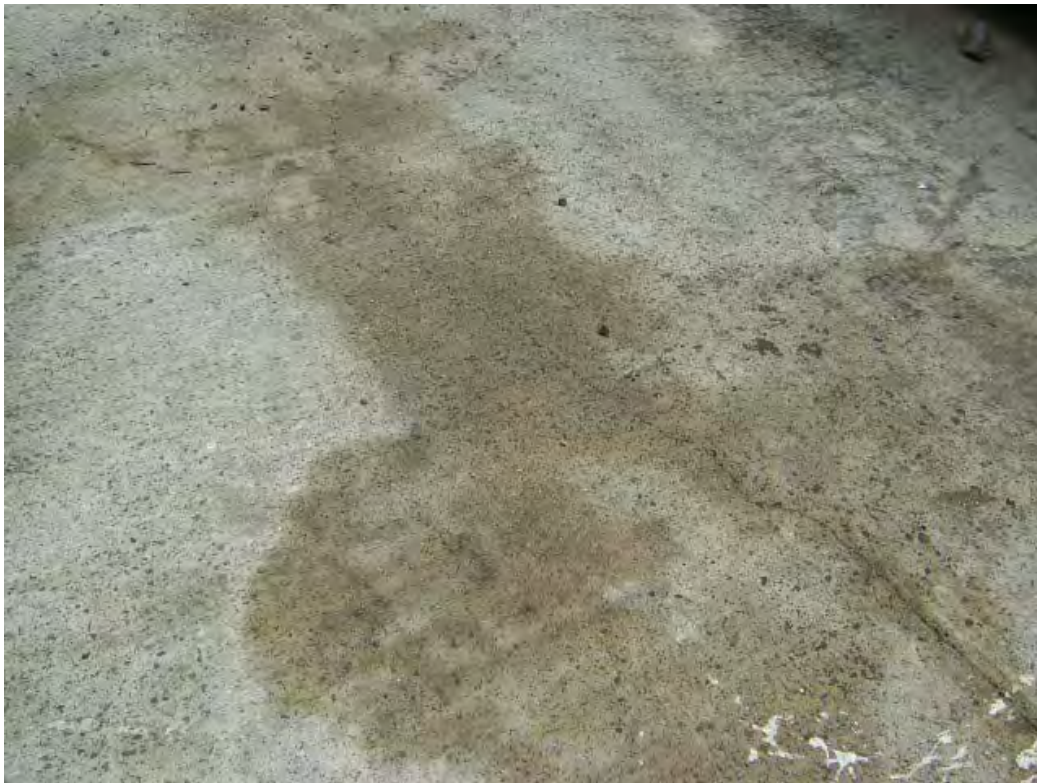
Oil Stained Concrete Floor in Engineering & Maintenance Area
