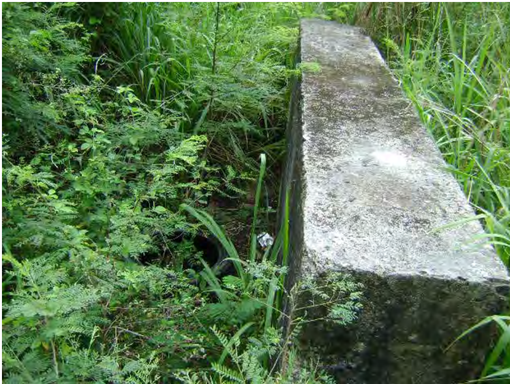
Concrete Structure in Area of Former Above Ground Fuel Storage Tanks on Tract 04-104
