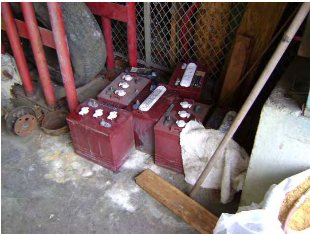
Automotive Batteries & Stained Concrete Floor in Engineering & Maintenance Area
