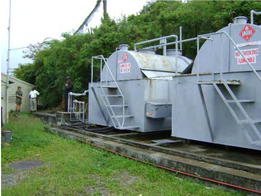
Above Ground Fuel Storage Tanks at Marina Facility
