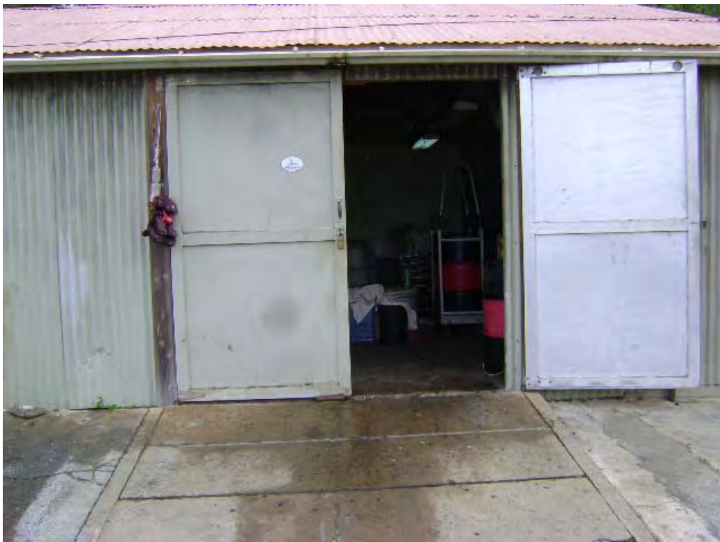
Oil Stained Pavement Near West Building of Marina Facility
