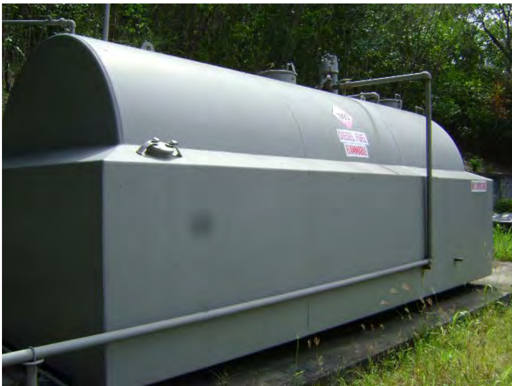
Above Ground Diesel Fuel Storage Tank for Emergency Generator
