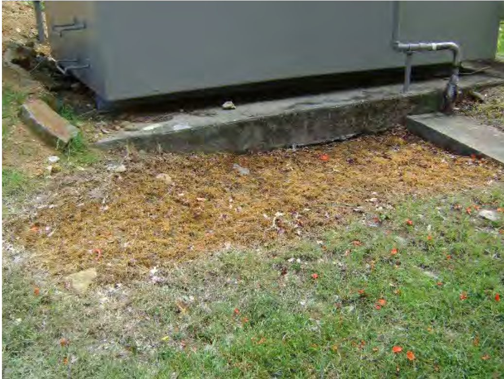
Distressed Vegetation & Fuel Impacted Soil Near Gasoline Fuel Tank North of Generator Building
