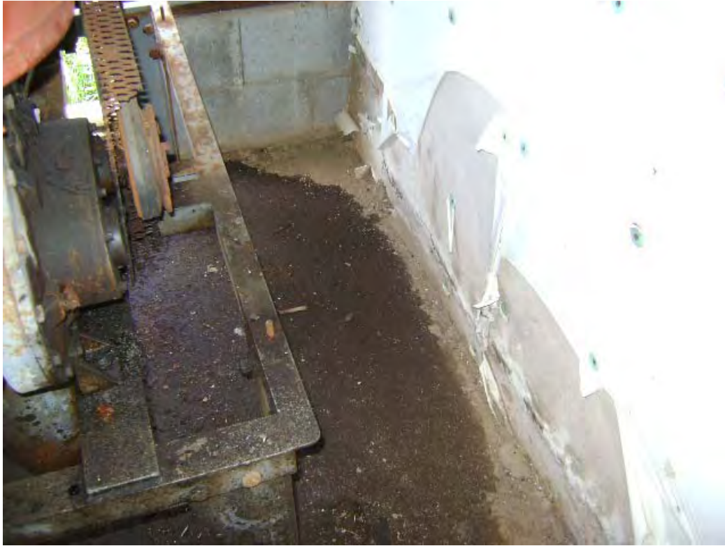
Oil Stained Floor Near Pump in Building at Wastewater Treatment Plant
