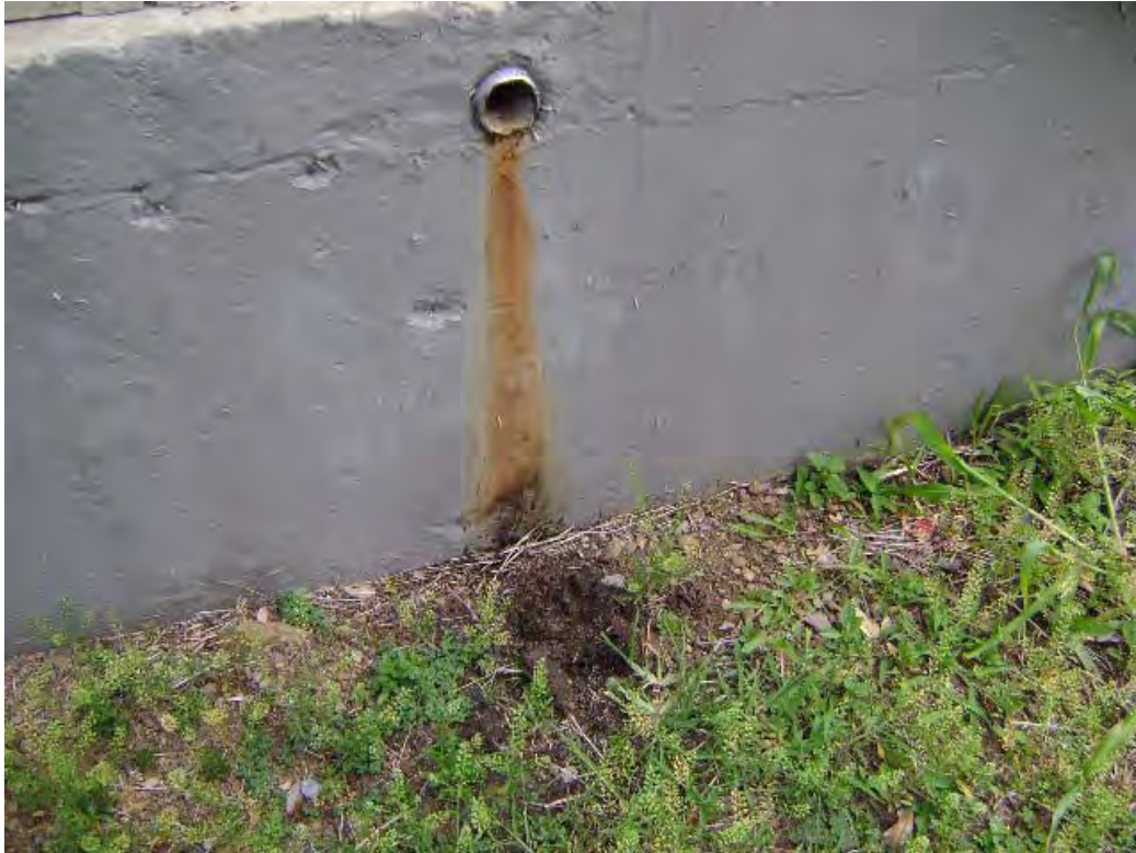
Oil Discharge From Floor of Emergency Generator Building to Soil Outside Building
